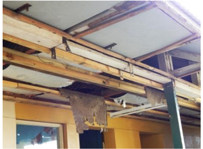
Hospital ceiling and eaves damage still to be repaired
